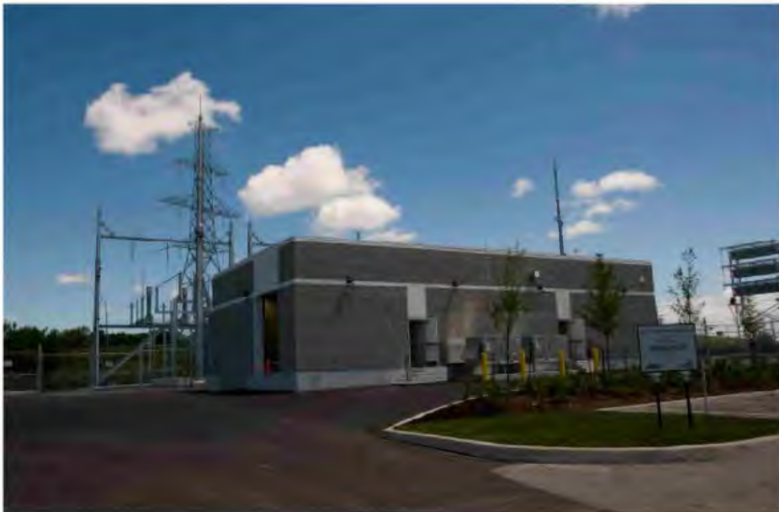
Construction of the Fabro Transformer Station in Markham was completed early in 2010. It is one of 11 transformer stations owned by PowerStream that are directly connected to the provincial transmission grid.
